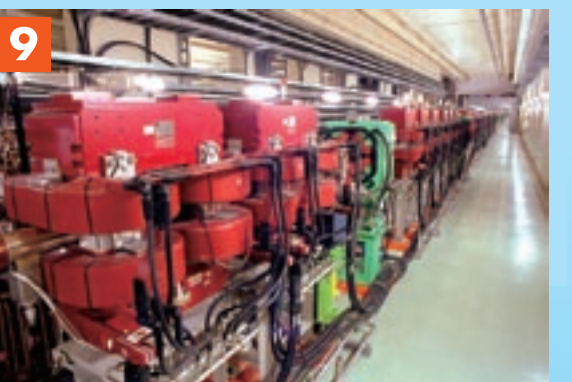
Wiggler magnet: This special magnet suppresses beam oscillations by taking advantage of, and strengthening the effect of, the beam's own damping mechanism called "radiative damping."
