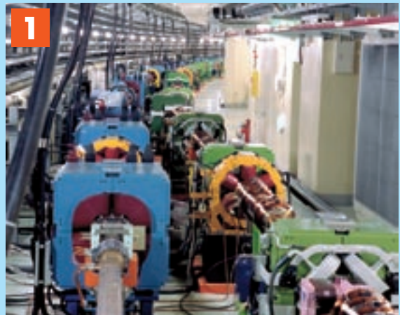
Electromagnets in the arc region: Electromagnets guide beams in a circle, and are one of the critical accelerator components. More than 2,000 electromagnets of various types are employed.
