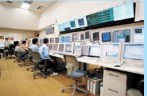
Control room: Accelerator scientists control KEKB's many pieces of equipment from the central control room. Many monitors are lined up to display the current status of the accelerator. The central control room also controls equipment at sub-control rooms located around the ring.
