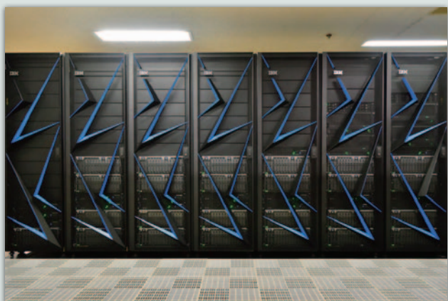
IBM Elastic Storage Server GL4C (25.5PB)
